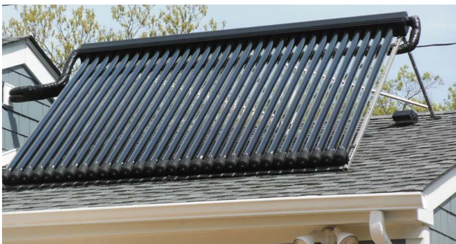
Two 30-tube evacuated tube panels provide solar thermal water heating.
