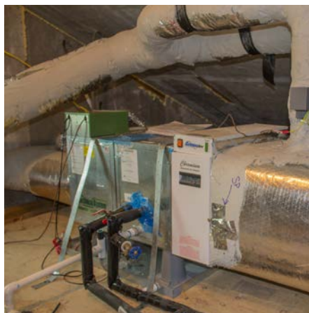
The air-to-water heat pump is installed within the conditioned space of the insulated attic.
