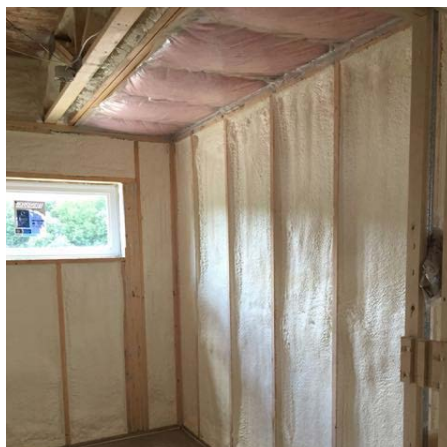
Closed-cell spray foam fills the exterior walls and cathedral ceilings of the home, providing insulation and air sealing.
