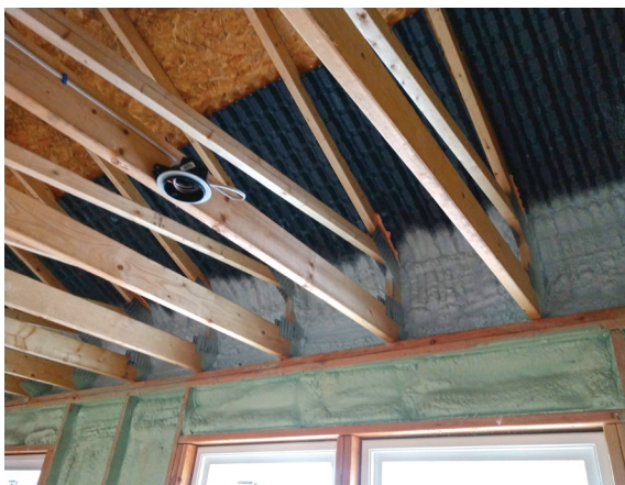
Walls are "flash" sealed with spray foam, which also seals the attic ventilation baffles to the top plates.
